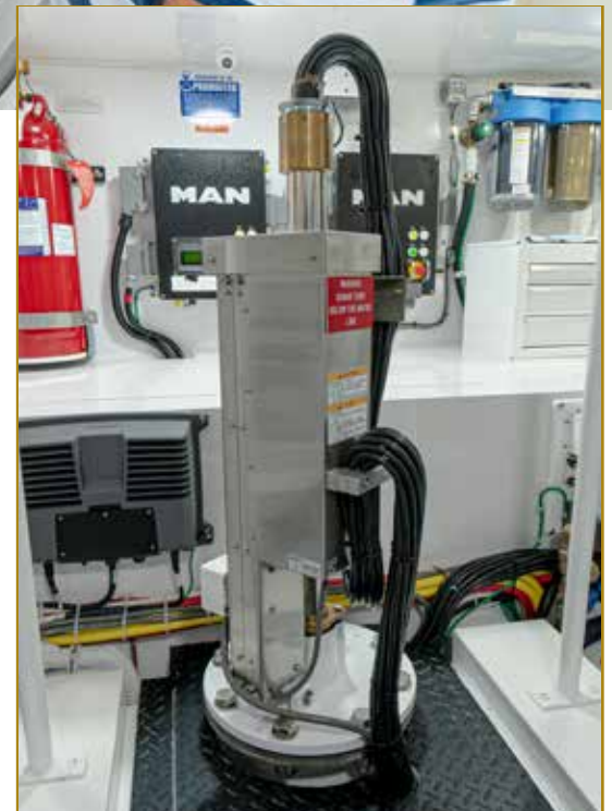
The Furuno system’s sonar tube installed in the engineroom.
